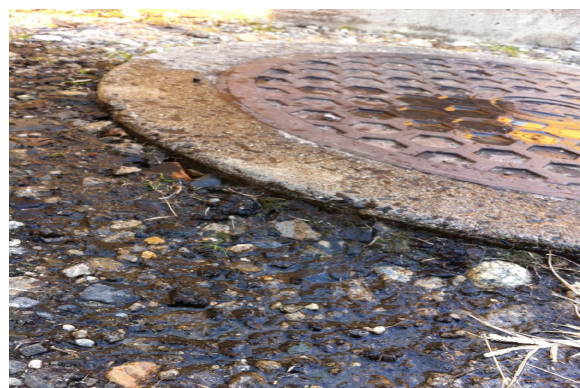
Fig. 3 Watering at the exposed natural base soil around a manhole in Fukumuro area
