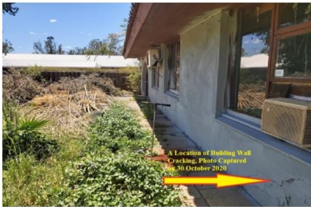
FIGURE 8: A LOCATION OF EXISTING BUILDING CRACKS
