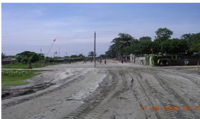
Figure 4: Sagufta Housing embankment preparation at Ch 4+150 in 2006, it was raised appx. 2.5 m from this surface to maintain 100 yrs ARI (1% AEP) during road embankment construction
