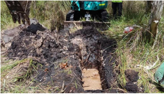
Figure 45: Photo 08. Soil collapsing into Test Pit location (TP7) and ground watertable encountered at 0.9 m depth
