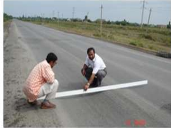
Figure 2: 70 mm deep rutting along wheel track, km 1+600, Source: from the project file
