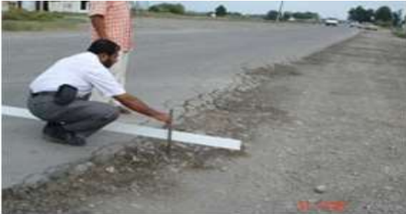
Figure 5: Shoulder erosion and edge failure at km 8+200, Source: from the project file
