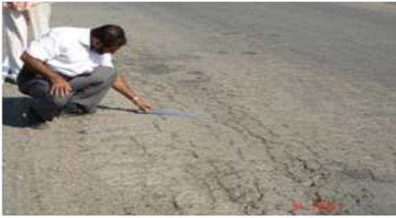
Figure 4: 3 ~ 15 mm wide crocodile cracks at km 7+700, Source: from the project file
