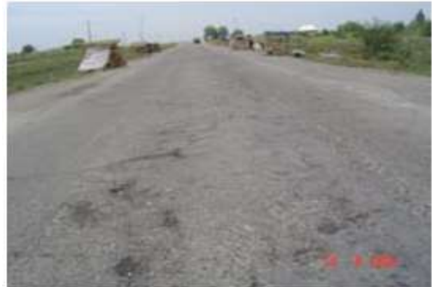
Figure 3: Cracked and undulated surface at Km 25, Source: from the project file
