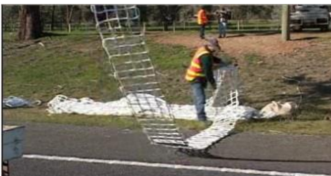
Figure 27: Installation of Rope net hooking between two poles, Possum and Fauna crossing (ladder type), Source: Nationwide Netmakers Pty Ltd
