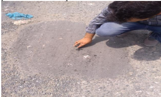
Fig.2 Pavement softness due to temperature
